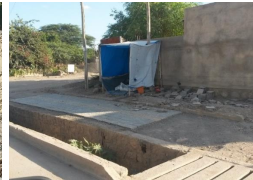
Pavement works in progress (East-West southern road). Sidewalks are taken into account in new road projects.
