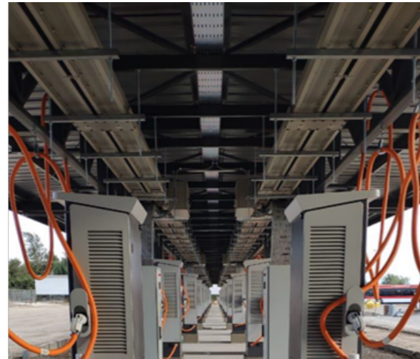
Figure 8. Example of how charging infrastructure can be built into the roof to lessen space requirements.
