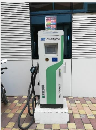
Nagpur City – Public electric cars charger
