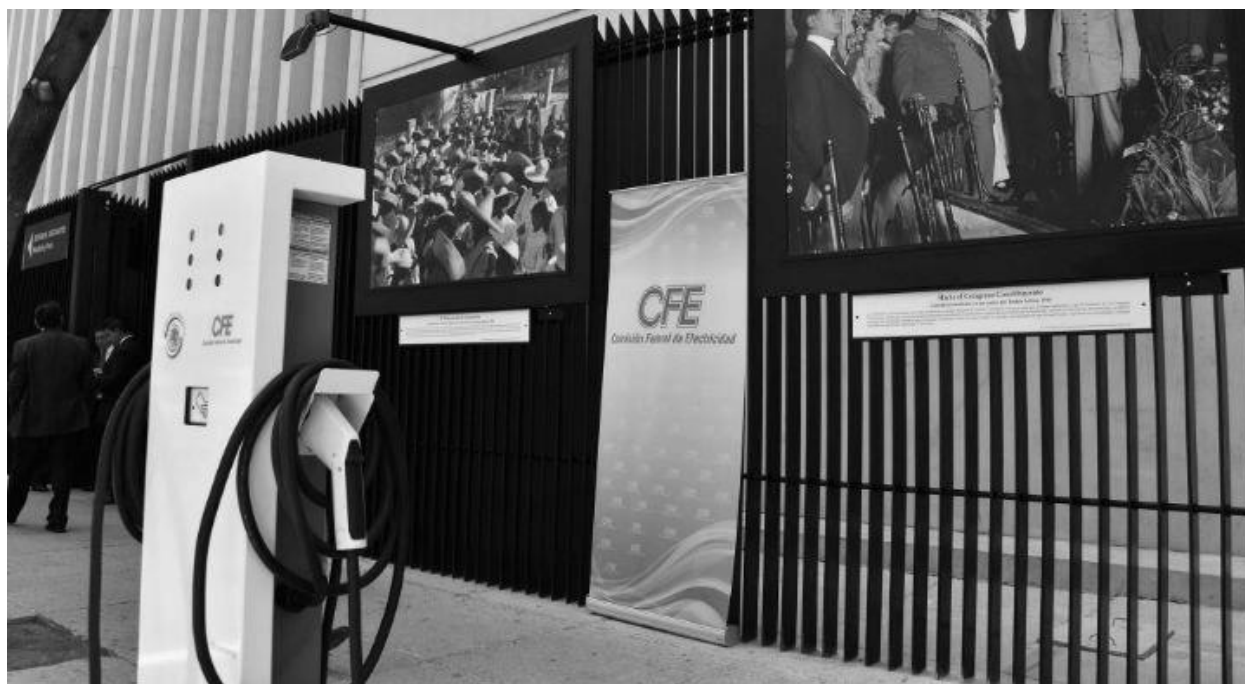
Figure 7. Photograph of a public charging unit installed by the Federal Commission of Electricity in Mexico [107]
